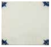
Field Tile Cracked (With corner designs)
